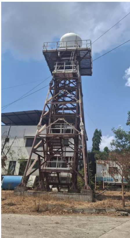
4. Fig. Radar Facility, Water Filtration Plant, Kalyan Dombivli Municipal Corporation (KDMC), Mumbai
